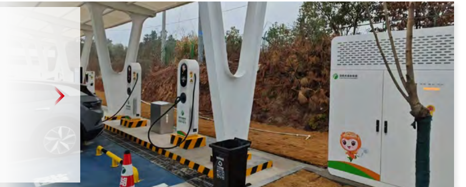
Hunan Expressway Full Liquid Charging Station
