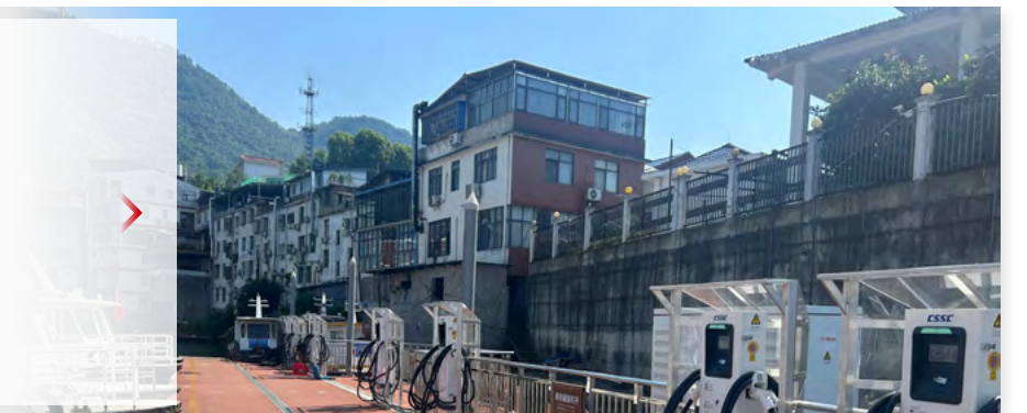
Wuhan Resort Area Onshore Charging
