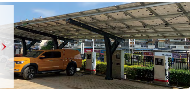
State Grid PV-ESS Charging & Discharging Test & Demonstration Pilot Station
