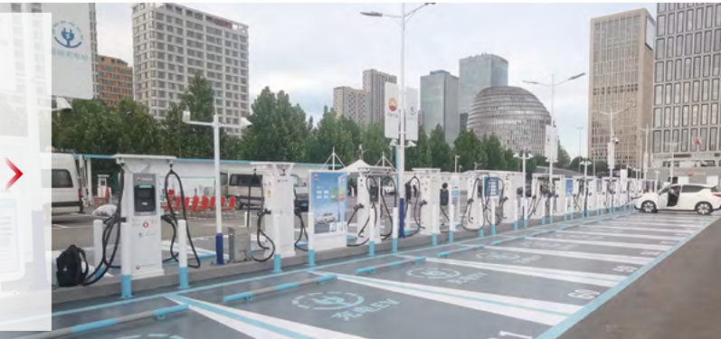
PetroChina PV-ESS Integrated V2G Charging and Battery Swap Station Global First
