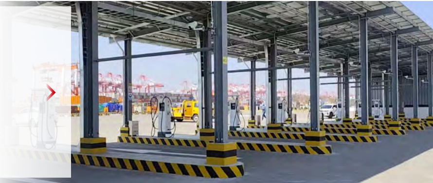
Shanghai Port Charging Station
