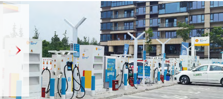
Shell (China) Public Charging Station
