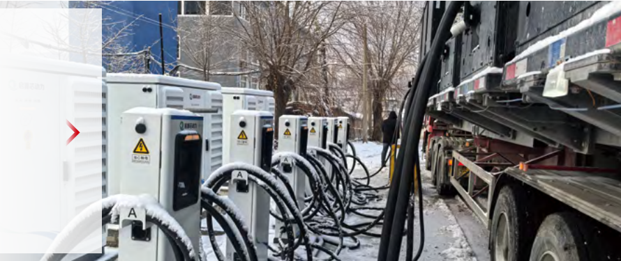
Liaoning -30°C ~40°C Heavy-Duty Truck Charging Station
