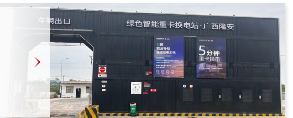
Auto Group A Battery Swap Station
